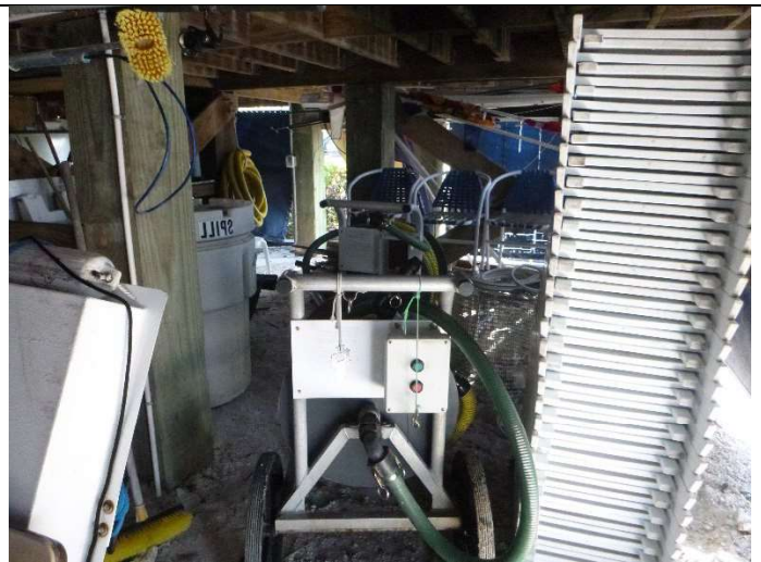
26. View of pump out equipment
