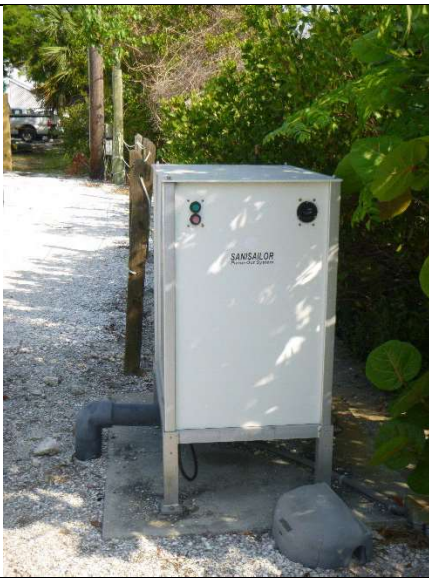
31. View of pump out station
