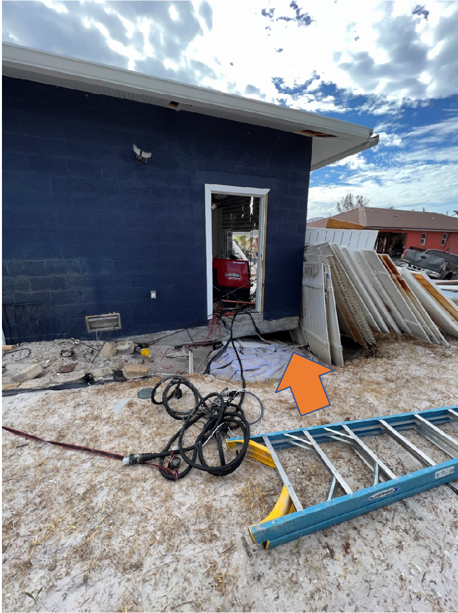
The above picture shows a side view of the shed. While it does have foundation washout, the building otherwise seems to be in adequate structural condition.
