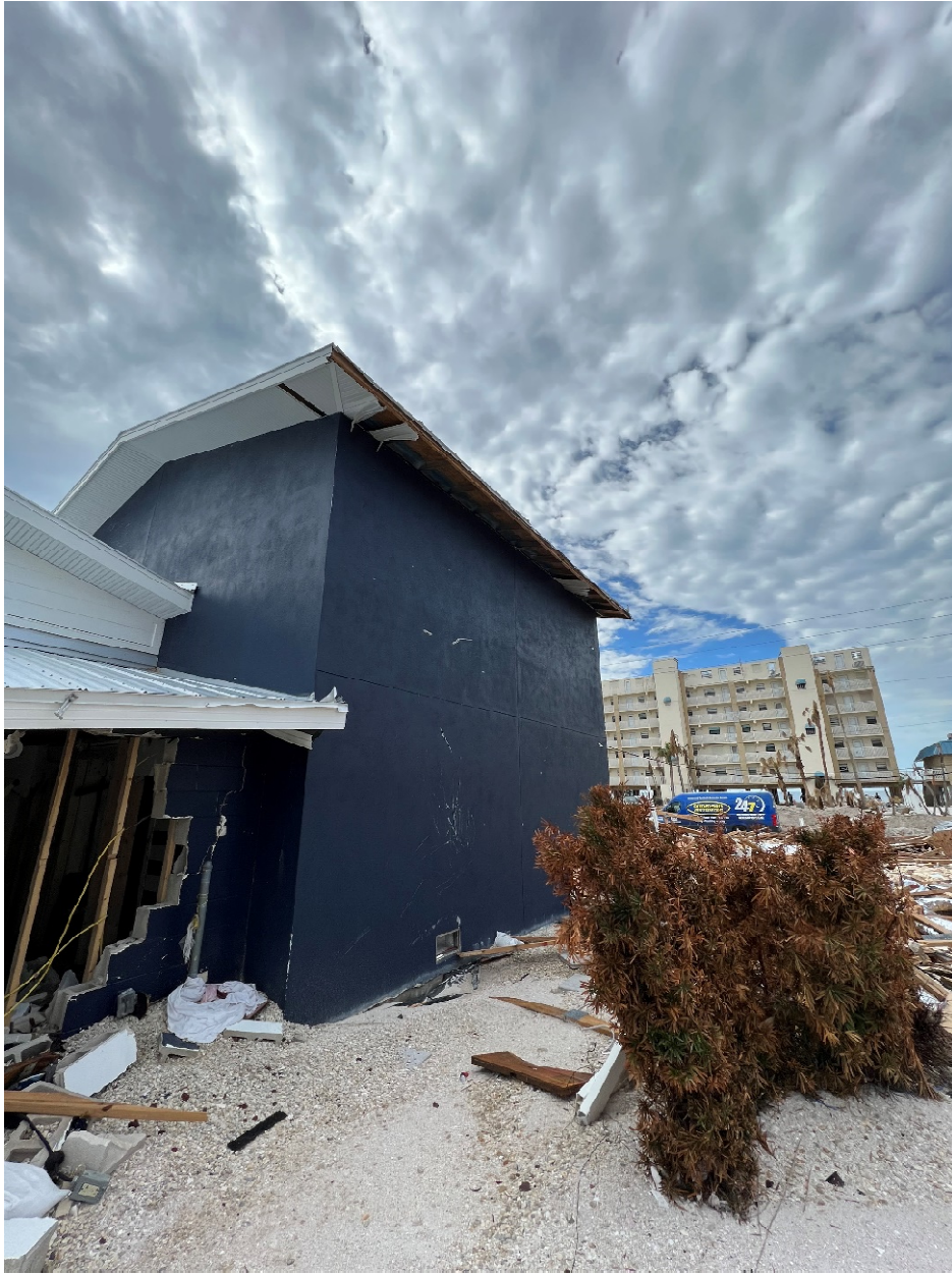
The above picture shows the back left view of the garage and the destroyed house behind it. The garage appears to be in adequate structural condition, while the house is not.
