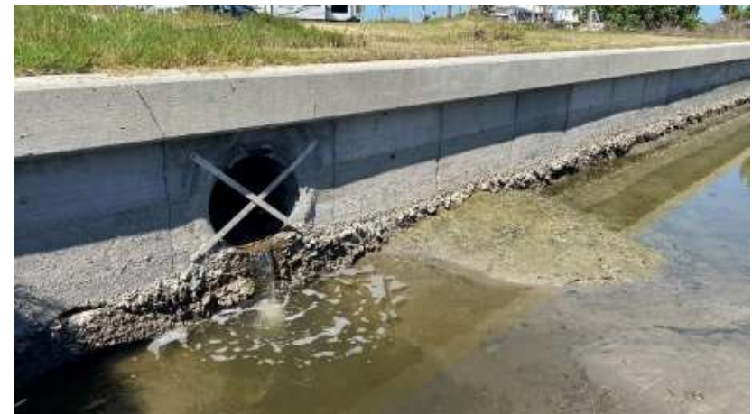
Figure 4-16. Outfall of the Stormwater System
