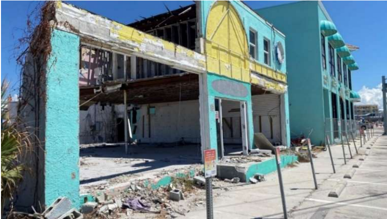
Figure 3-16. Damaged Commercial Property Near Times Square
