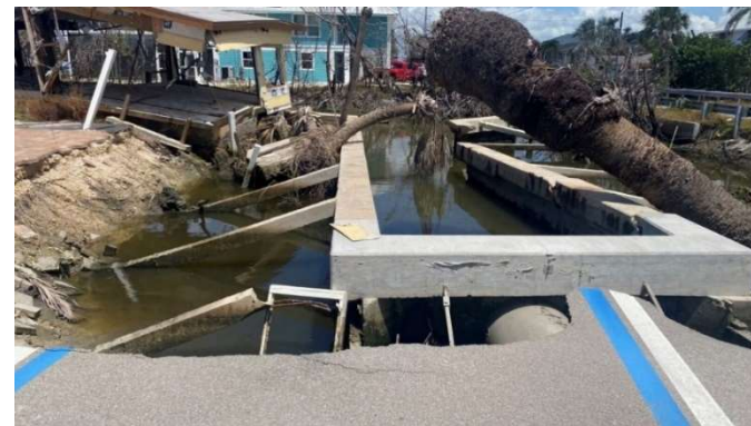
Figure 3-17. Damaged Seawall and Building Along a Canal
