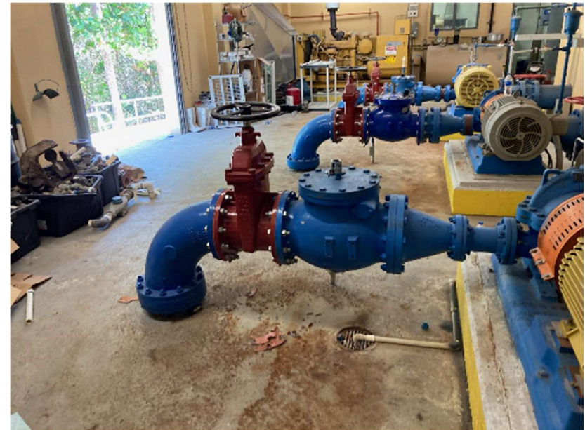
Figure 4-20. Booster pumps at the South Pump Station facility.-
