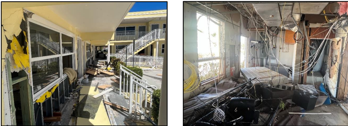
Figure 3. Post Hurricane Ian Photos
