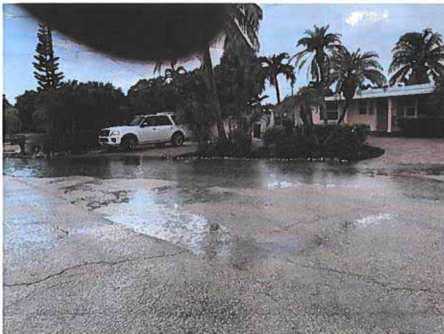
Ponding across cul-de-sac after barrier removal – entire cul-de-sac ponds
