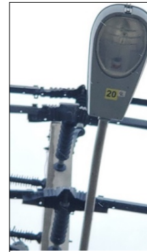
Figure 1 - Existing HPS luminaire on Estero Boulevard
